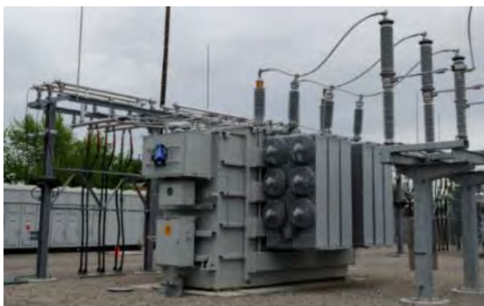
Substation power transformer
