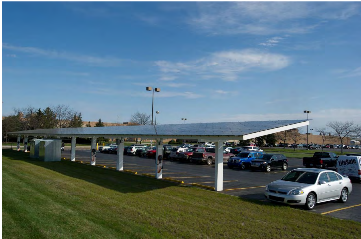
DTE industrial customer solar array and EV chargers
