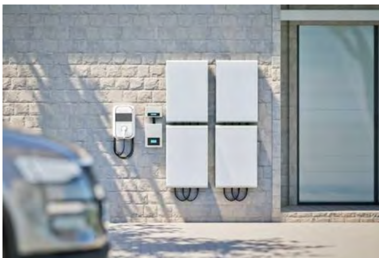
EV charger and energy storage
