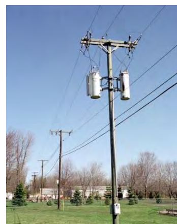
Overhead regulator on pole
