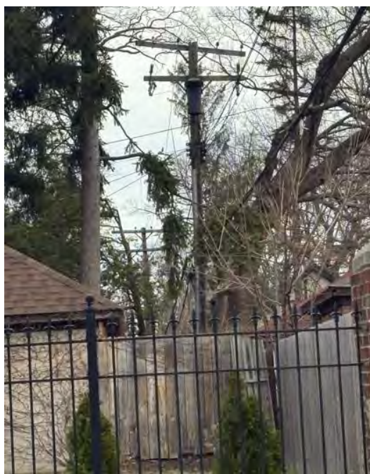
Legacy 4.8 kV rear-lot construction in Detroit
