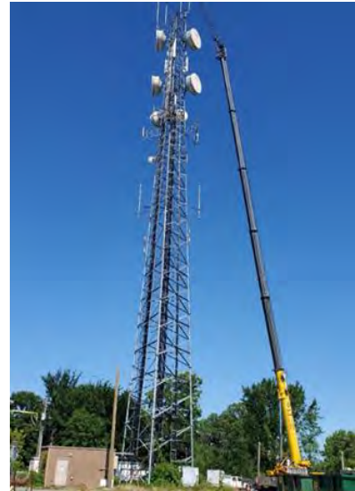
Wireless communications tower
