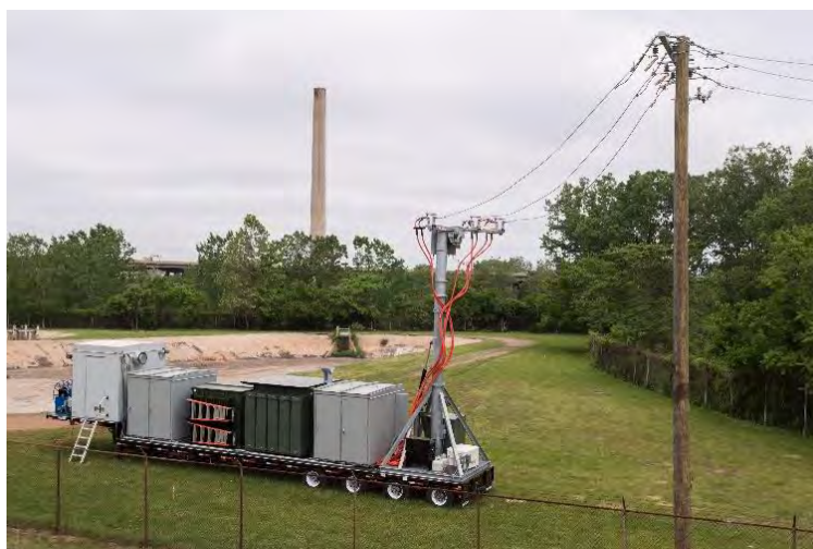
Portable substation trailer
