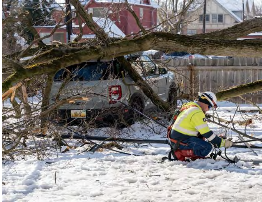
Storm restoration – downed secondary wire
